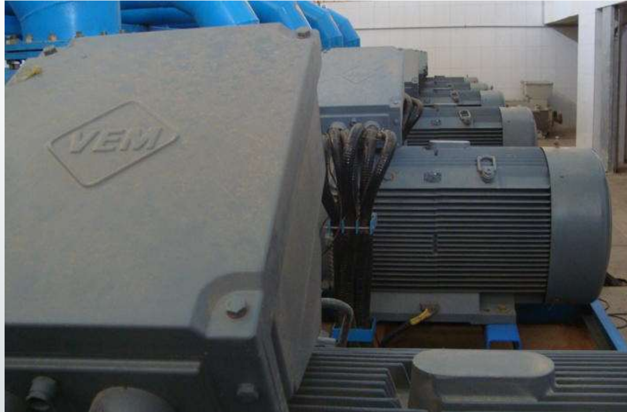
VEM motors- Gavshan water transfer project 110 KW to 355 KW, 1500 RPM, 2009
